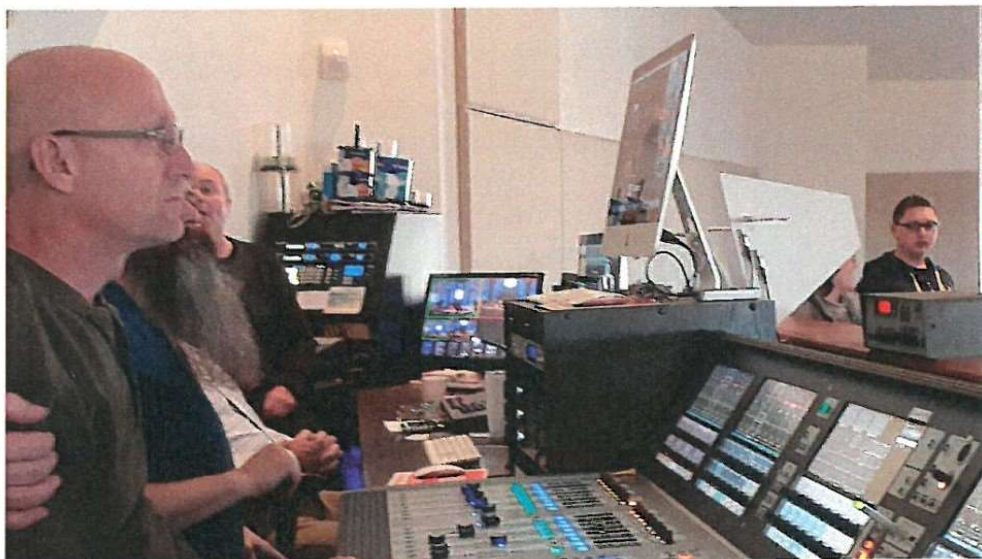
A portion of the sound and video console at Blue Valley Baptist Church. The live streaming equipment has its own room!
